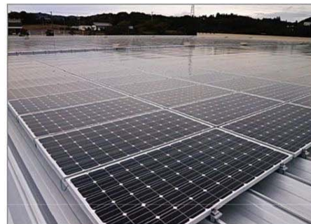
Project : Super Center PLANT Shima Branch Purpose : Commercial facility Completion : 2013 Area : Mie Prefecture Numbers of Panel : 3,808 Capacity : 1,142 KW
