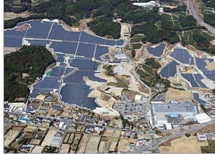
Project : 25th Makinohara Jitoho Solar Power Plant Purpose : Solar Power Plant Completion : 2016 Area : Shizuoka Prefecture Numbers of Panel : 65,408 Capacity : 19,546 KW
