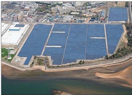
Project : CENERGY Mega Solar Edobashi Power Plant Purpose : Solar Power Plant Completion : 2014 Area : Mie Prefecture Numbers of Panel : 37,380 Capacity : 7,500 KW
